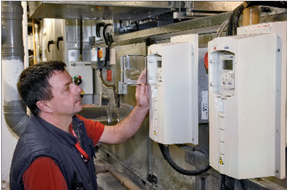
ABB standard drives for HVAC control the fans for the air conditioning system serving the two buildings that comprise the stadium's Quadrant expansion project.
