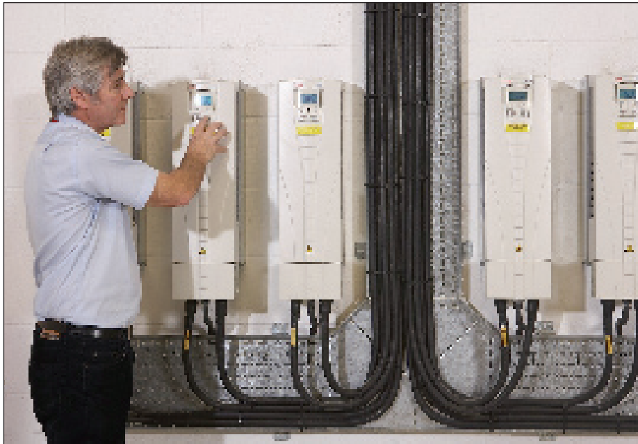
Maintenance costs were reduced through fewer motor belt breakages.
